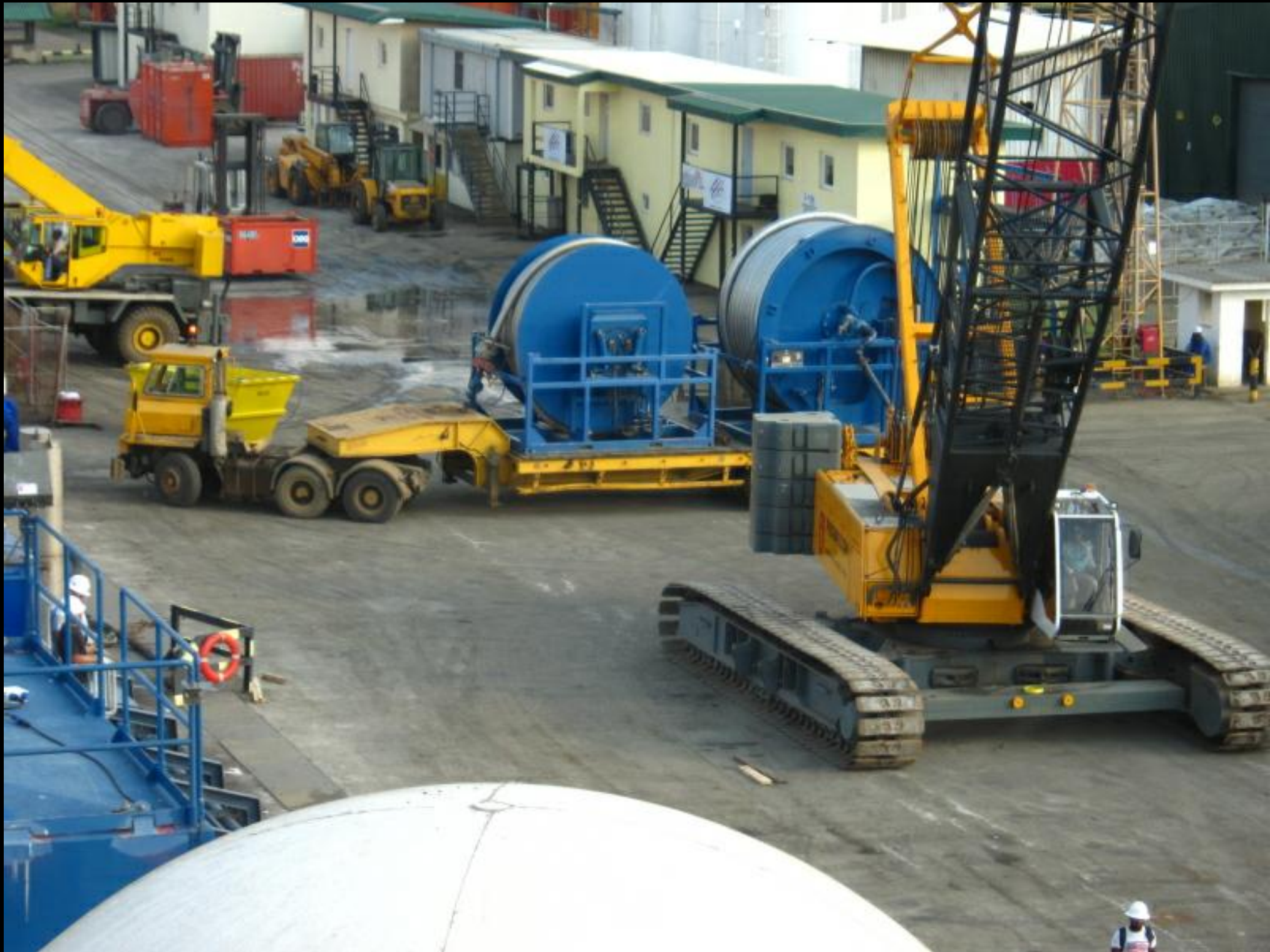
A reel of 3 inch coflex high pressure tubing and a reel of 4 inch were the last two pieces loaded to complete the frac plant.
