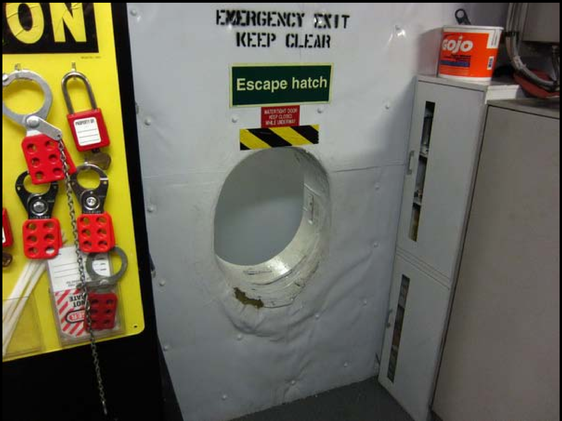
This escape hatch from the ECR is not meant for large people. The hatches on submarines are larger than this. It was fun going through it (and a real challenge).
