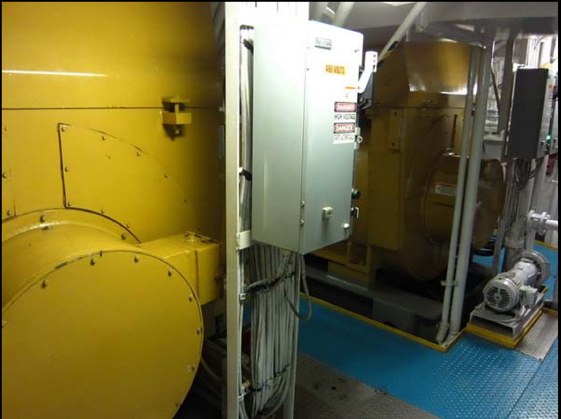
Here are two of the four main generators, each generating 1800 KW of power at 480 Volts.
